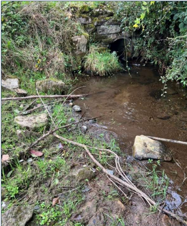
Plate 4-38. A representative image of the pipe culvert at the upstream survey extent at GC 9
