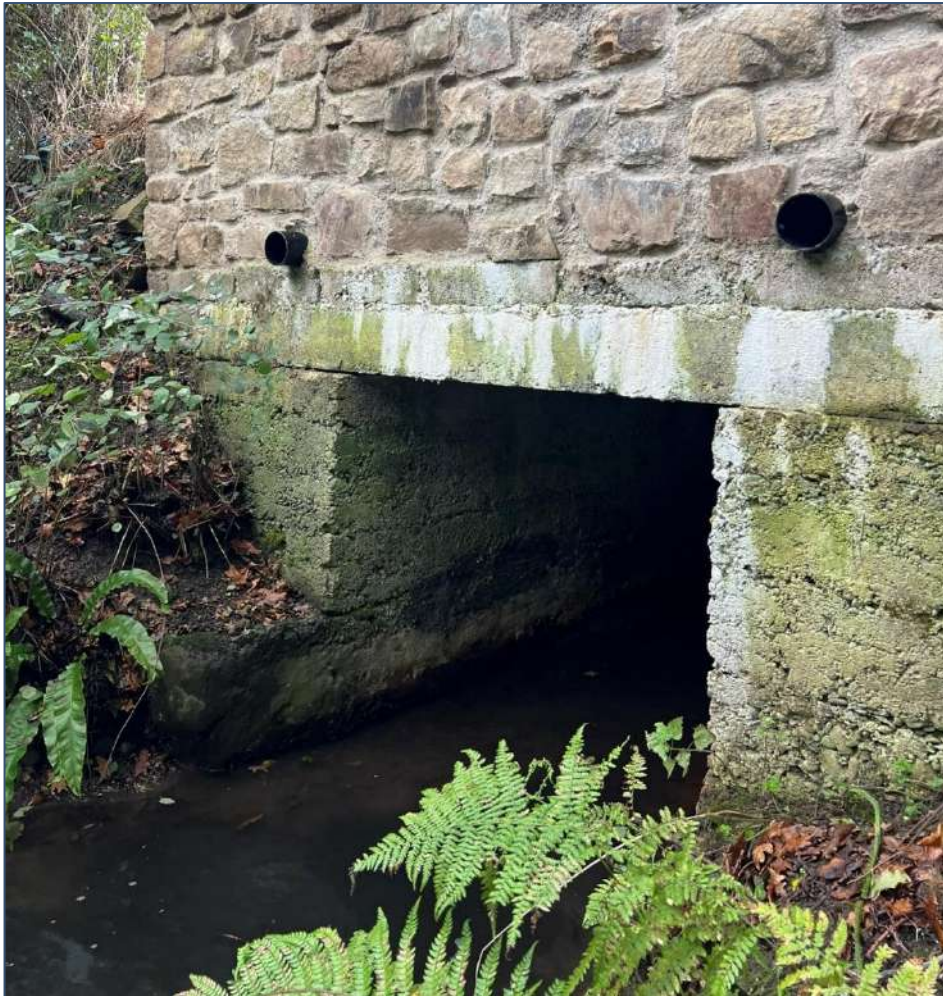
Plate 4-55. A representative image of the bottomless concrete culvert at survey location GC 19
